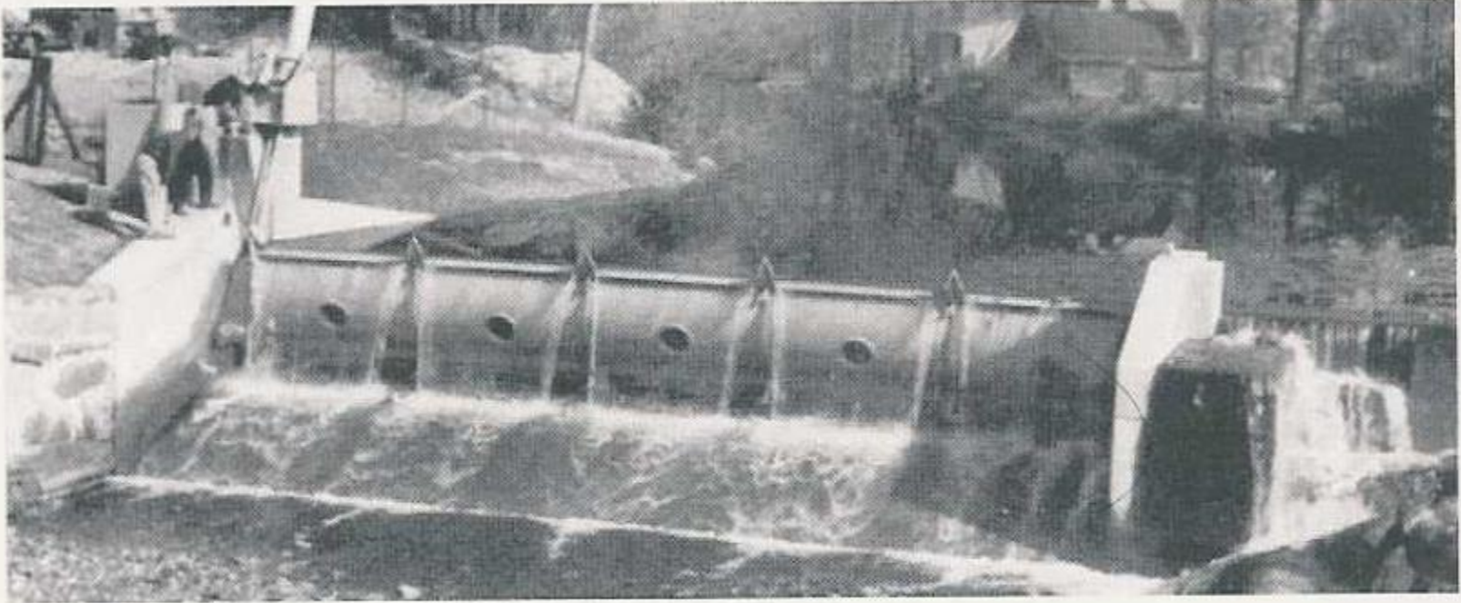
Fig. 2.6 Downstream view of a flap gate with nappe breakers (RODNEY HUNT)
